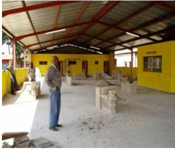
The interior of a partly finished 'health centre' by a Chinese Company in Lusaka, Zambia
